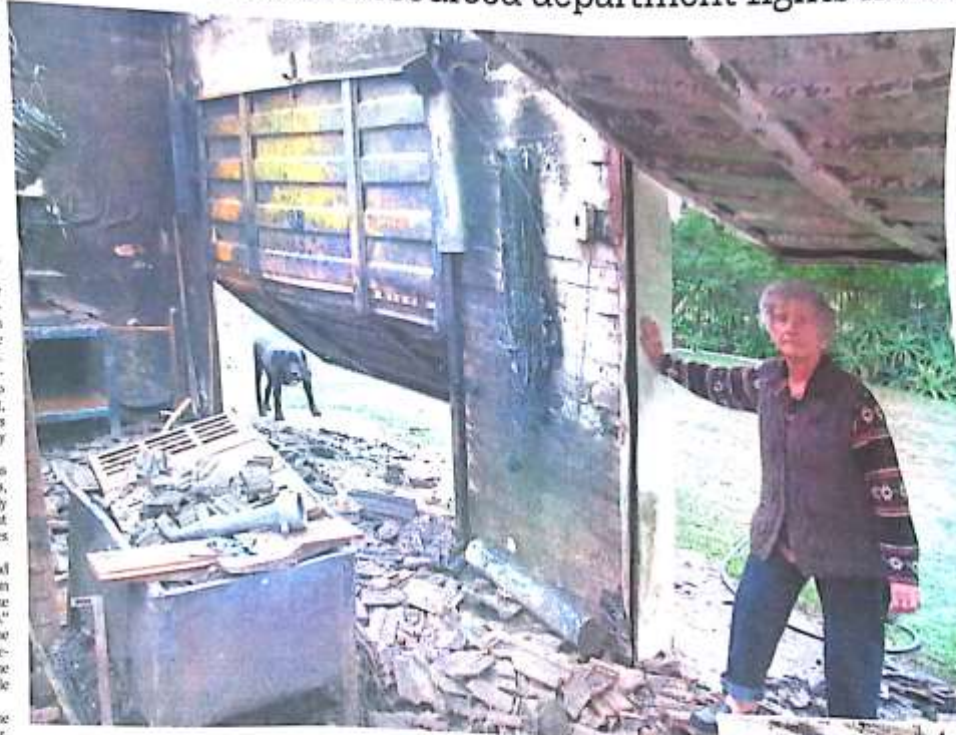
LEFT: Lois Cross surveys the damage after part of her family's Ashburton home was damaged in a fire yesterday morning.
